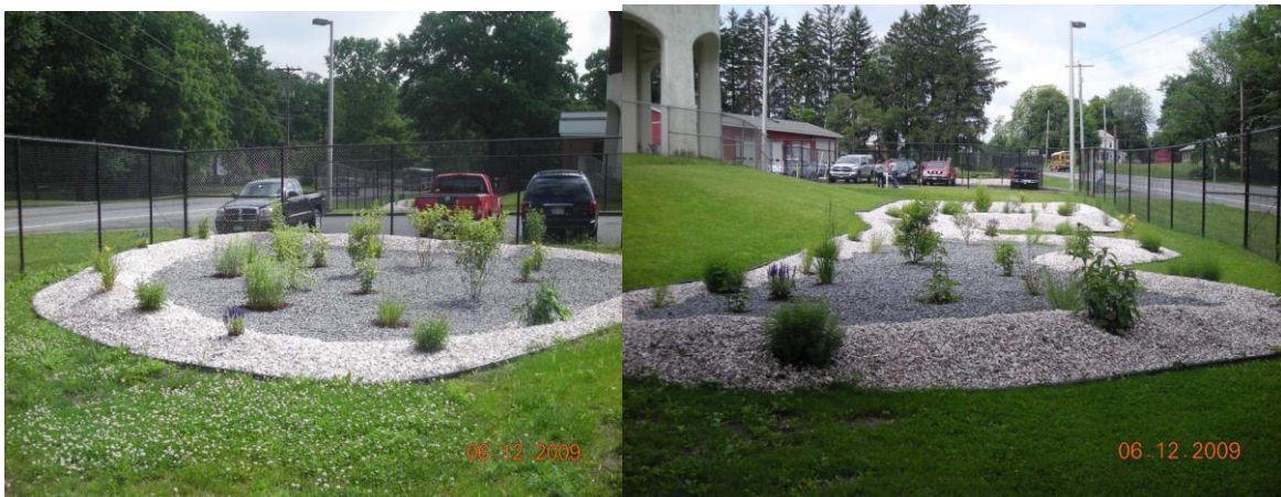
Rain gardens installed at the City of Newburgh Water Treatment Plant (Images courtesy of Orange County Soil & Water Conservation District)
